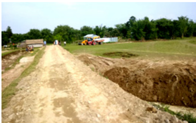
Figure 7.2. Construction of bunds in eastern part of 1st plot in RARS, Gossaigaon
